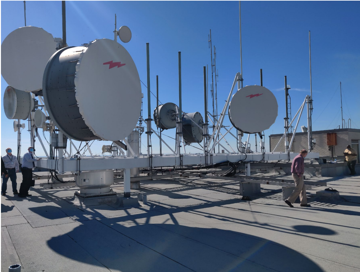
Existing Microwaves (Non-MARTA) on Ravinia Tower
