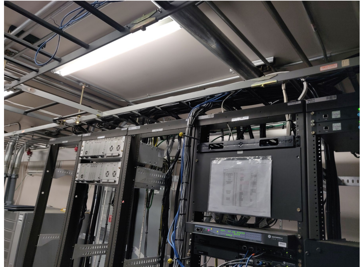
Network Room inside Ravinia Tower (Non-MARTA)
